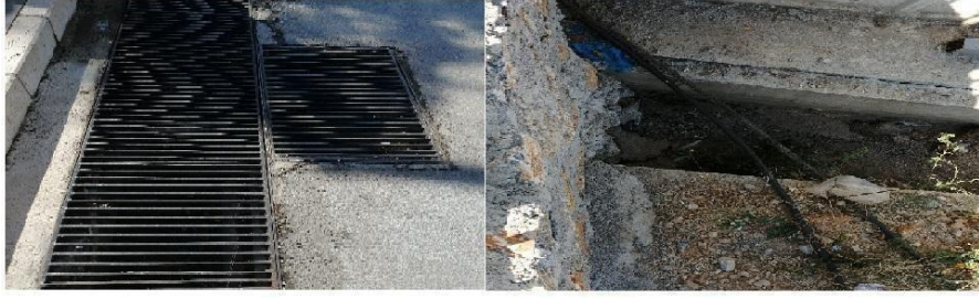
Figure 18: The Drainage System Separating the Rain Water from the Sewage on the Main (Kötekli) Campus
